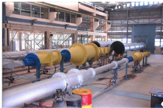
High Speed combustor test facility
